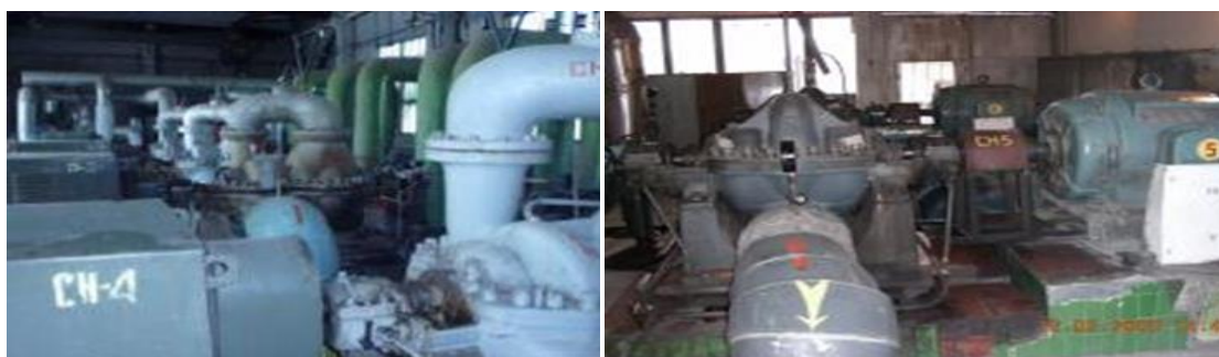
Figure 3.5: Circulation Pumps at DH Pump Stations 1 (Left) and 4 (Right)
