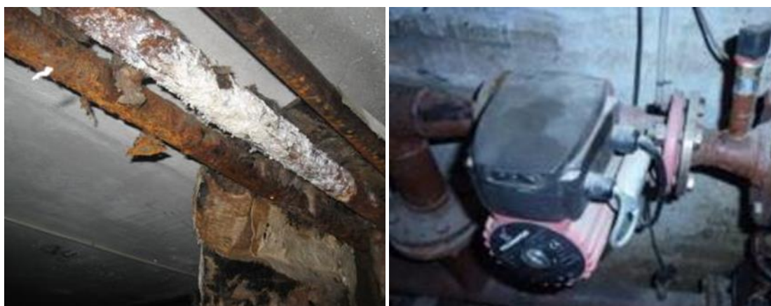
Figure 3.6: Worn-Out Hot Water Pipelines (Left) and Flow Regulation at a Substation (Right)
