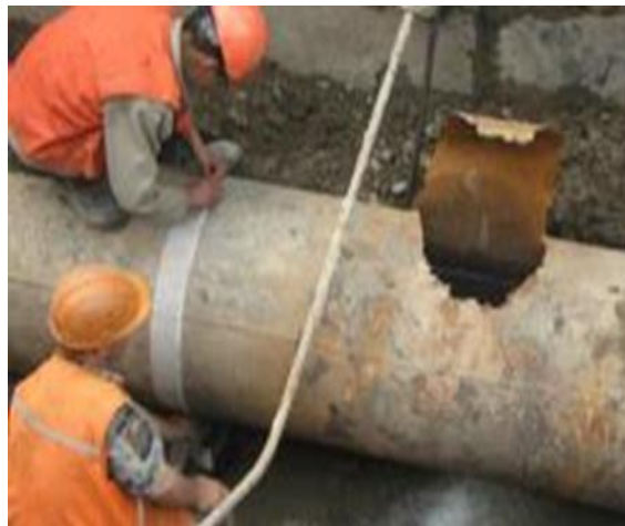
Figure 3.4: Picture of Damaged CHP 1 DH Transmission Pipeline
