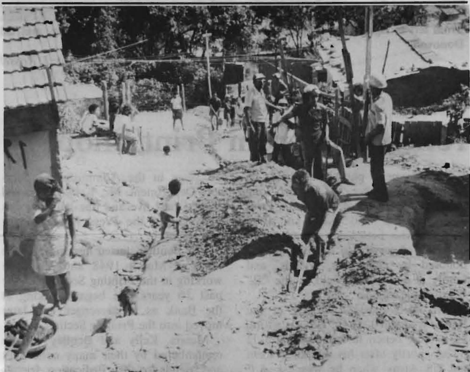
Local volunteers dig ditches for a water supply project in Minas Gerais state.
