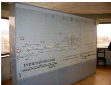
Central Dispatcher Control Panel, Georgia
