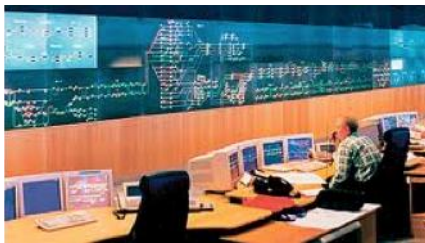
Train Control Center
