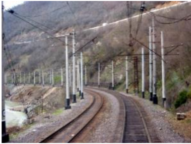
3kV-DC Overhead Catenary, Georgia
