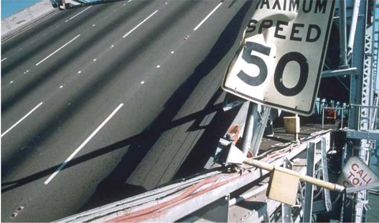
Loma Prieta earthquake damage on Bay Bridge, California, in 1989.
