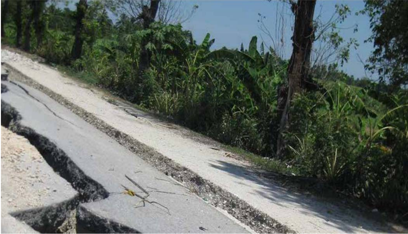
Earthquake-damaged road between Port-au-Prince and Léogâne has failed, but is still in a functioning state. It is now at risk of complete failure during rainy season as the subgrade is exposed.
