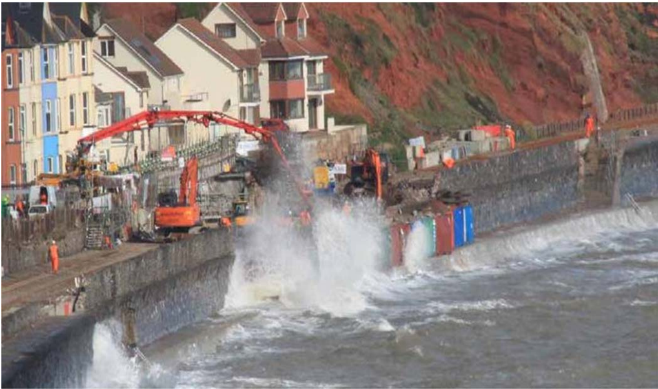
Pouring concrete to plug the hole in the sea wall below Sea Lawn Terrace at Dawlish, UK, on February 24, 2014.
