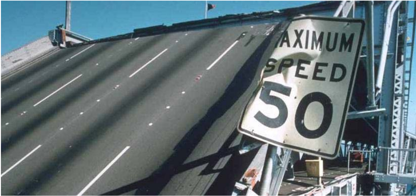
Bridge damage from the 1989 Loma Prieta earthquake in California.
