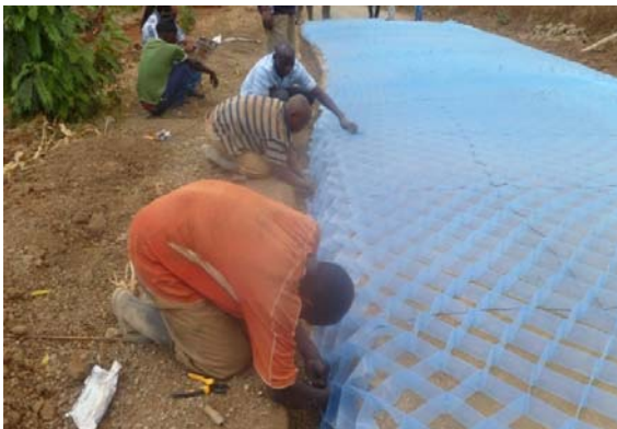
Geocells being installed as part of DFID's AFCAP (African Community Access Programme). Source: Roughton
