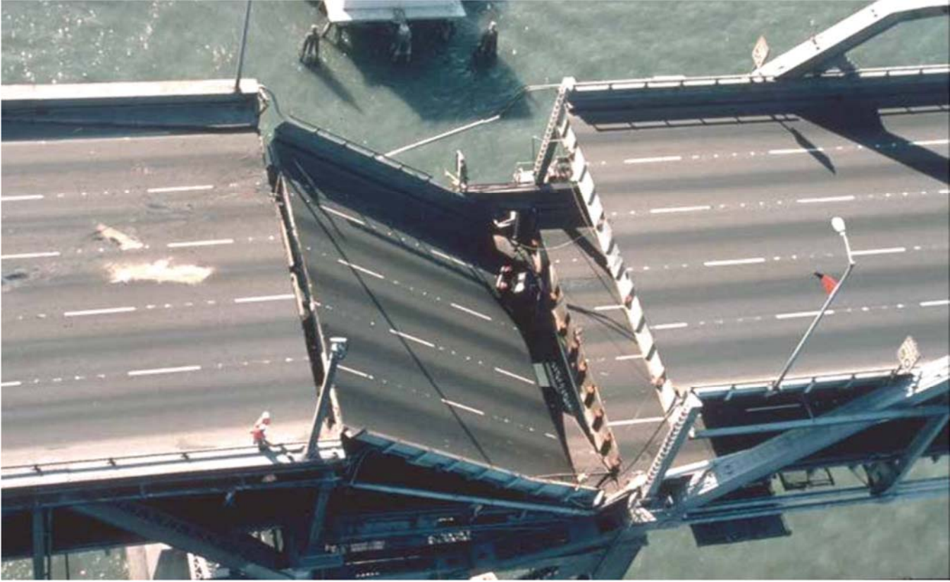
Loma Prieta earthquake damage on Bay Bridge, California, in 1989.
