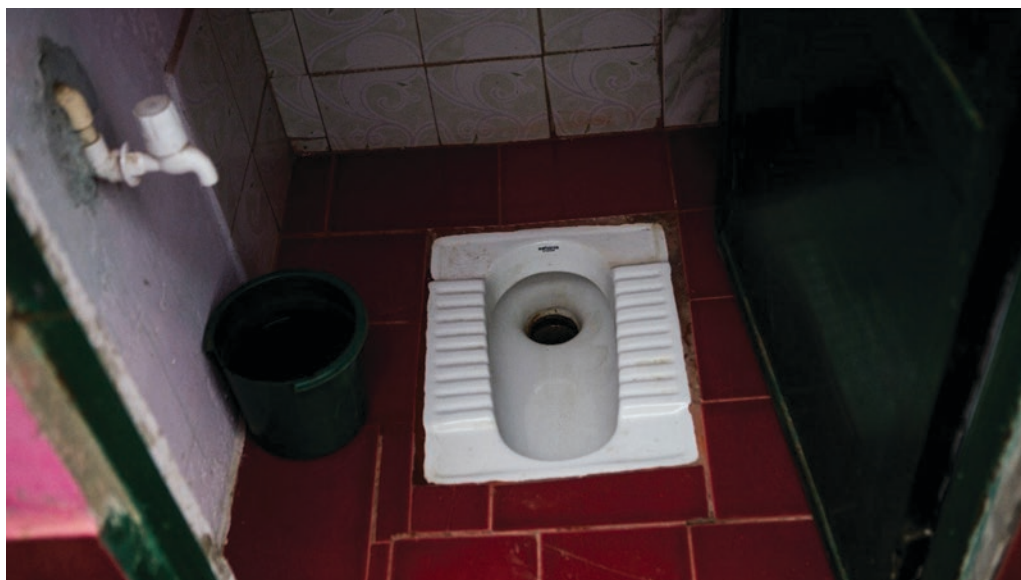
PHOTOGRAPH 16.2. Plastic Latrine Slab over Pit Latrine
