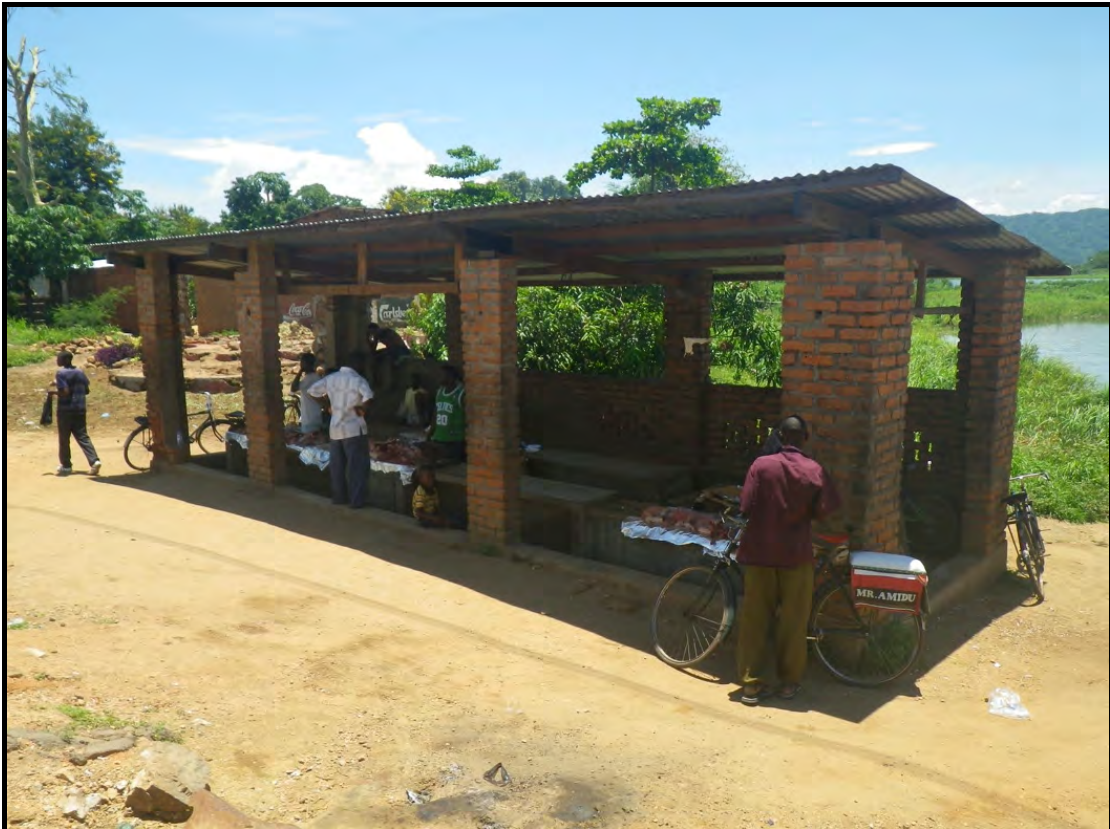
Figure 16. Liwonde Town Council Market Shelter- currently used as a butcher's shed on the Barrage approach, west bank.
