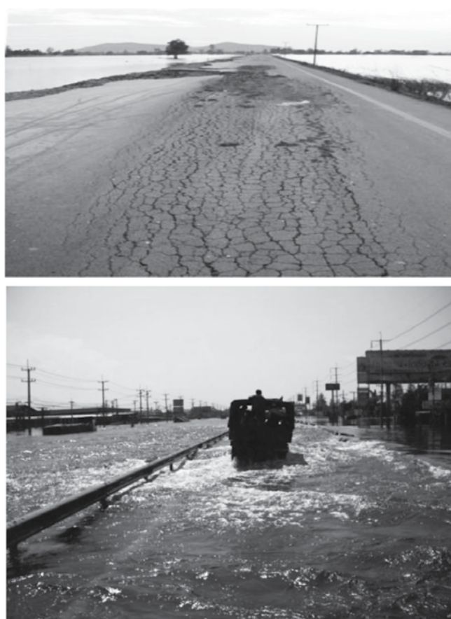
Figure 3.18: Damages from Flood on Road Infrastructure
