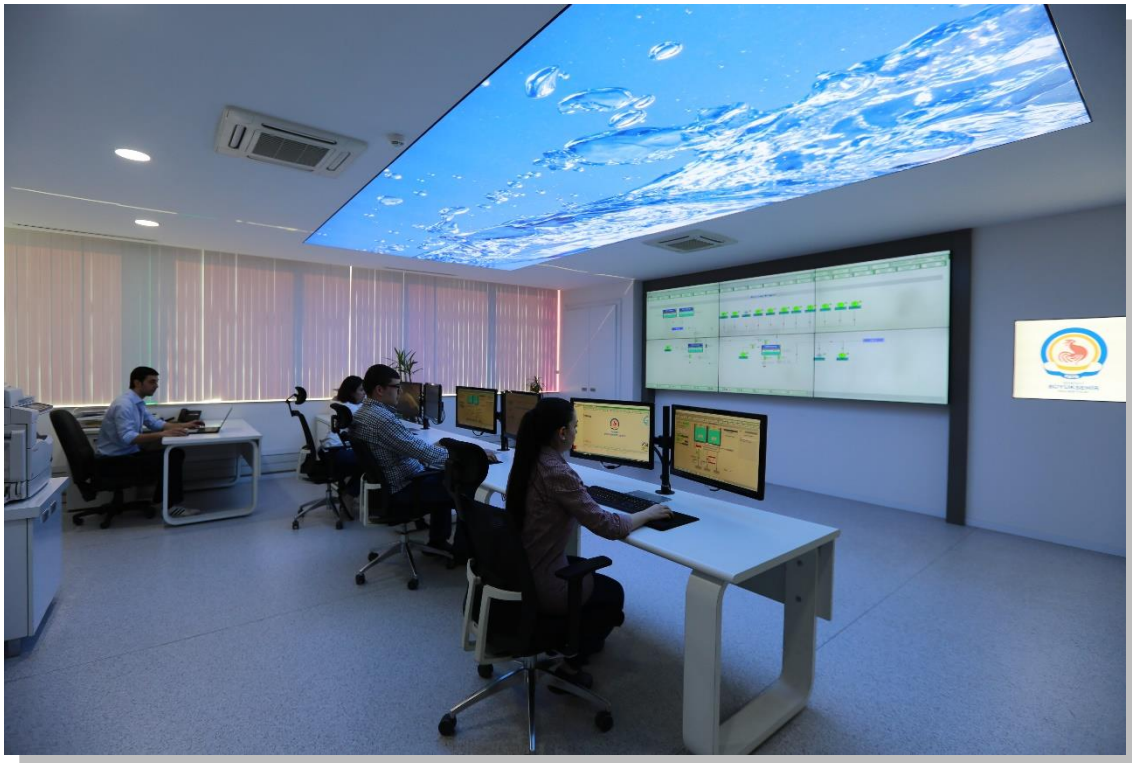
Figure 5.1. DESKİ SCADA Monitoring Centre
