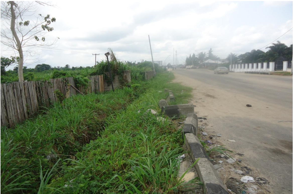
Plate 4.5: Poor Drainage System, Sapele/Warri Road, Sapele, Delta State
