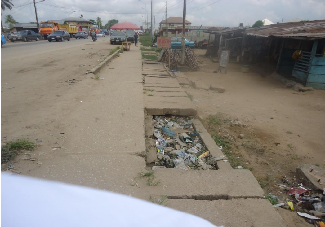
Plate 4.2: Accumulated Solid Waste on Drainage Channel, Okpe Road, Sapele
