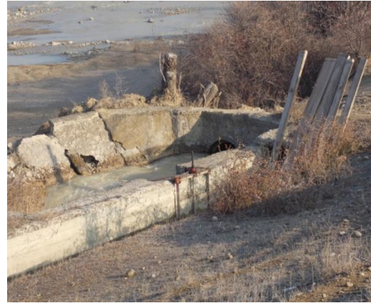
Water discharge well
