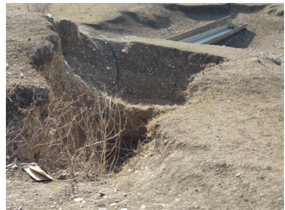
Erosion developed within artificially arranged pond
