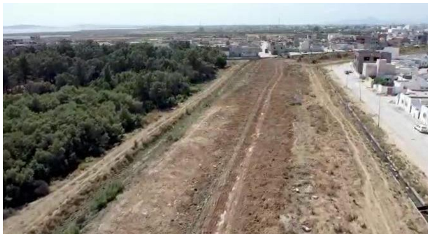
Picture A8.7 Fully underground TWW transfer system constructed under the Project, significantly reducing environmental and health risks to the community, and impeding recontamination along the line. Source: ONAS
