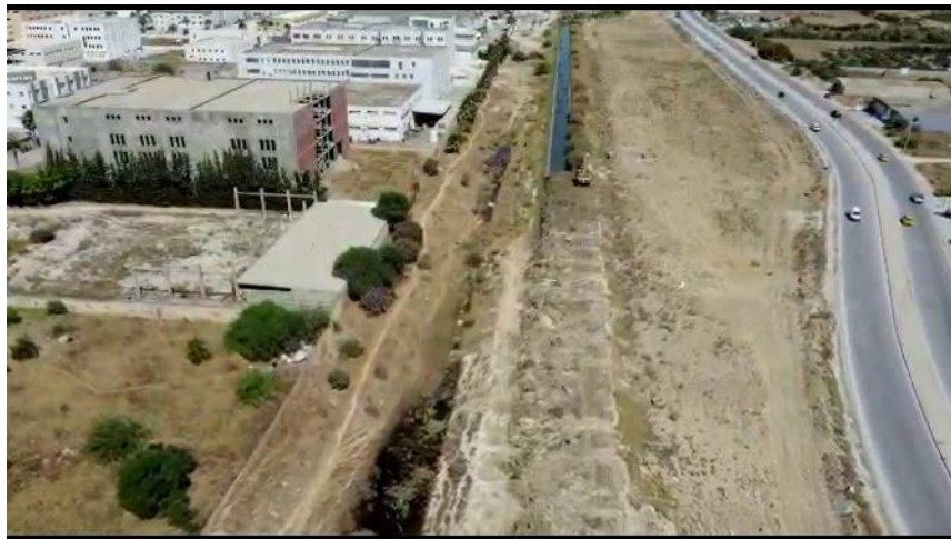
Picture A8.6 Open-air channel in the process of being decommissioned after the installation of the double underground pipeline. Source: ONAS
