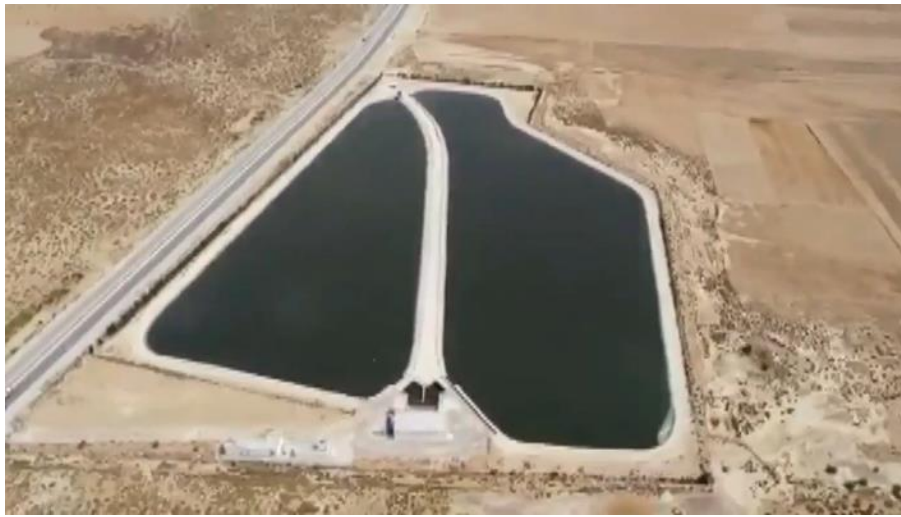
Picture A8.8 El Hissiene basin constructed under the Project, enabling TWW flow regulation for discharge to the submarine outfall and TWW storage for future reuse. Source: ONAS
