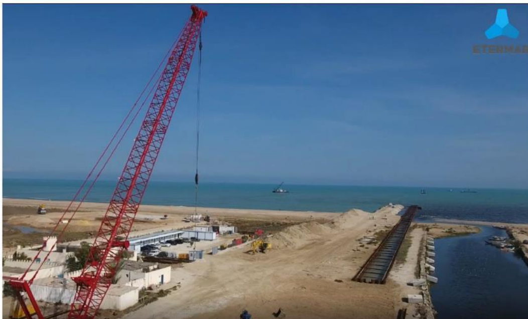
Picture A8.4 Installation of terrestrial portion of pipeline connecting to the submarine outfall. Source: ONAS
