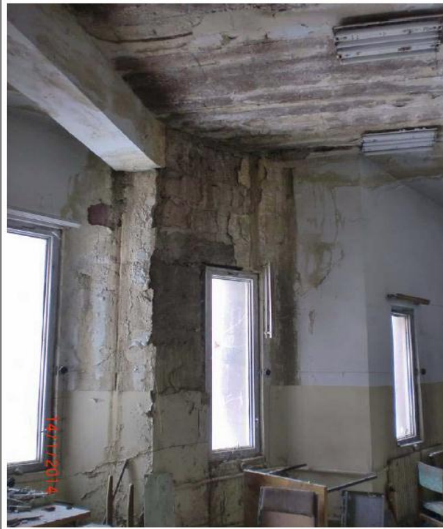
Extension 1. floor, Moisture damage and flaking on the ceiling and outer wall (Receiving Area 1)
