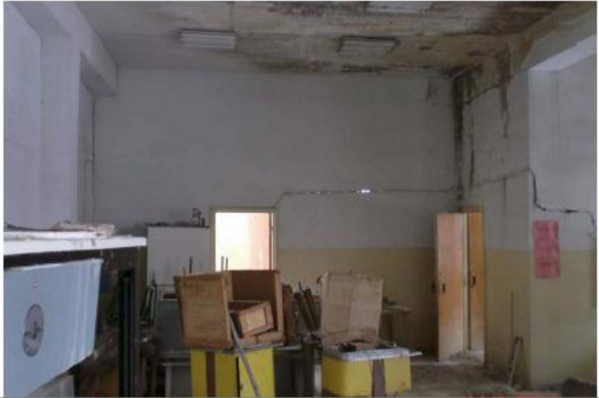
Extension 1. floor, Moisture damage and flaking on the ceiling (Receiving Area 1)
