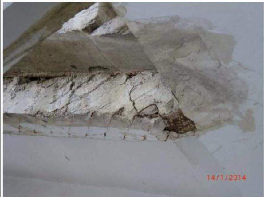
Main building 2. floor, Stairwell south side with damage on the staircase
