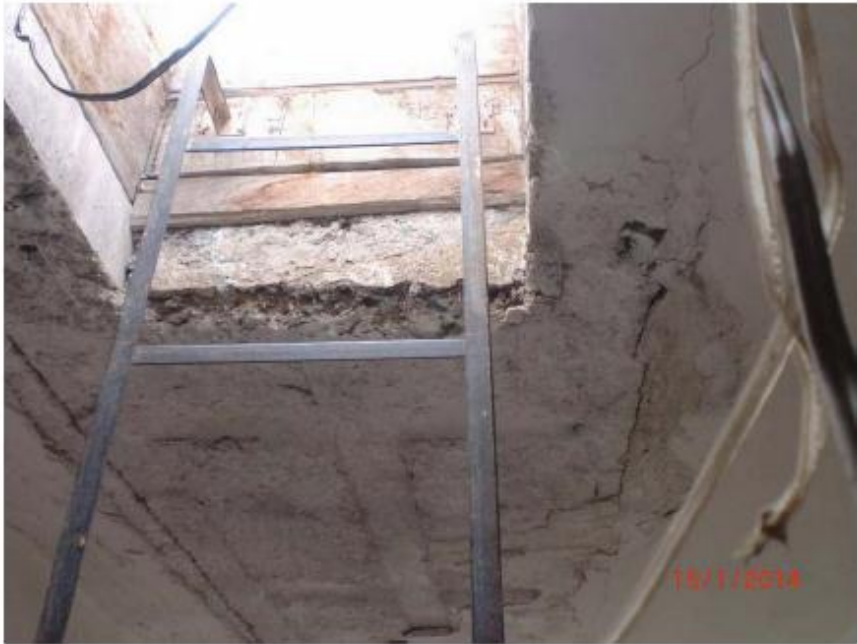
Main building 4. floor, Stairwell east side Roof hatch with concrete damage to the roof elements
