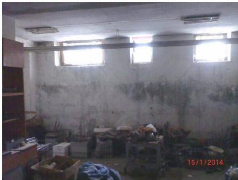
Main building basement, Workshop room street side with a damp external wall (Liquid Volume V3)
