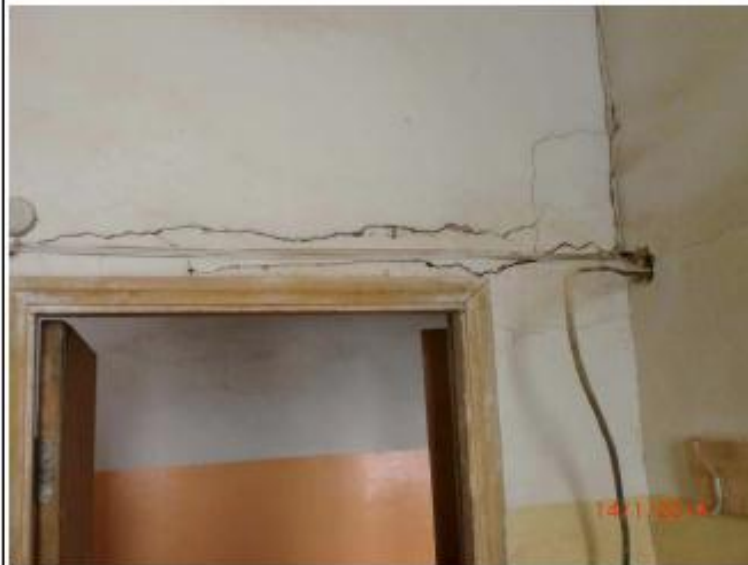
Main building 1. floor, Inner wall with subsidence on lintel of wood (Reception)
