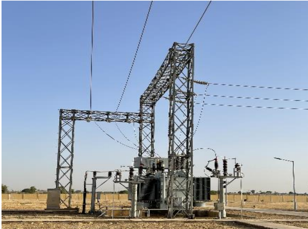
Picture: Malbaza Substation
