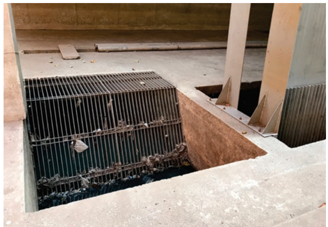
b. Primary treatment in wastewater treatment plant
