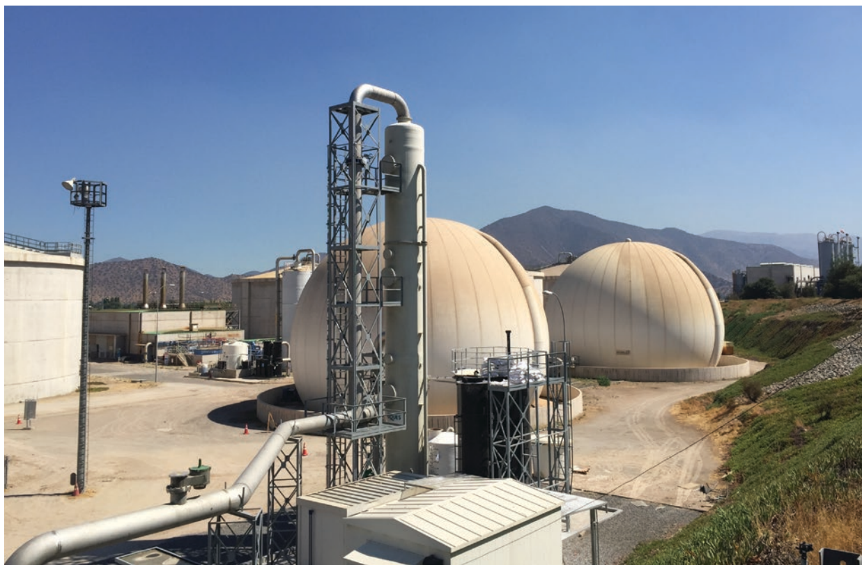
Biogas Holders at La Farfana Wastewater Treatment Plant. Source: Anna Delgado Martin / World Bank.
