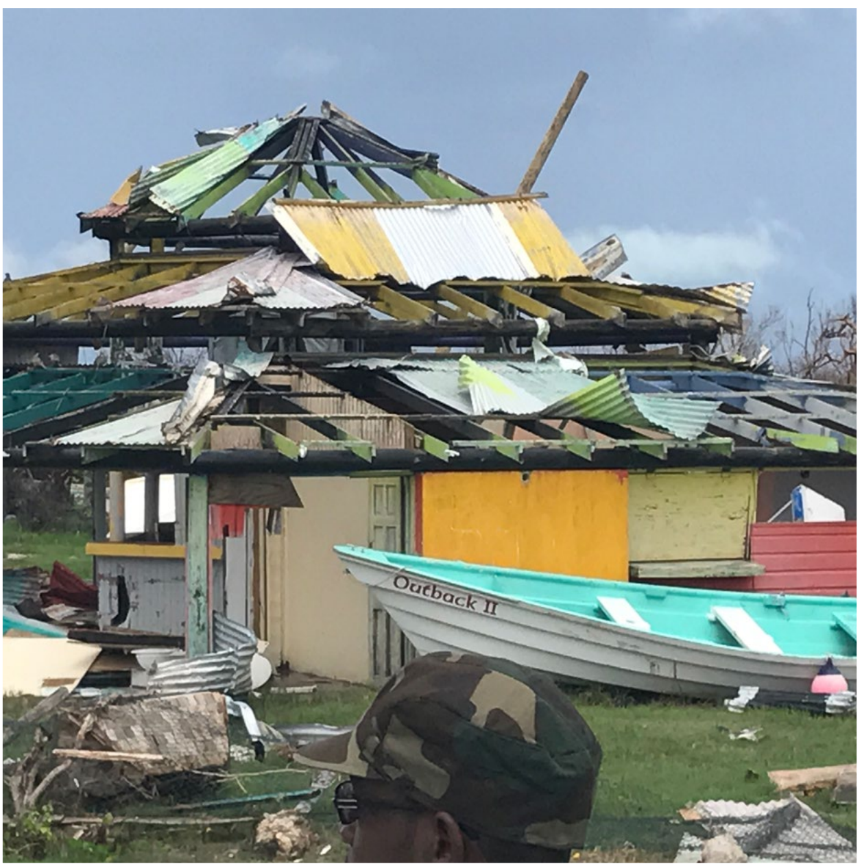
Destruction after 2017 hurricane in the Caribbean. Photo: GFDRR / World Bank
