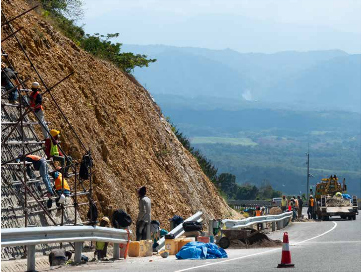
Photo: Building a retaining wall to protect against falling rocks on the Edward Seaga Highway in Jamaica. Debbie Ann Powell / Shutterstock.com
