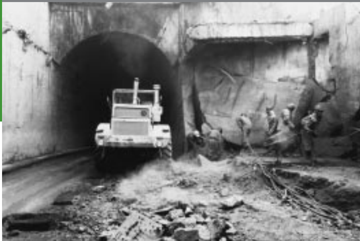
Through the Emergency Public Works and Community Empowerment Project in Afghanistan, work commences on the rehabilitation of the Salang Tunnel, the only entry point to Kabul for humanitarian aid and other goods as well as for refugees returning from the North.
