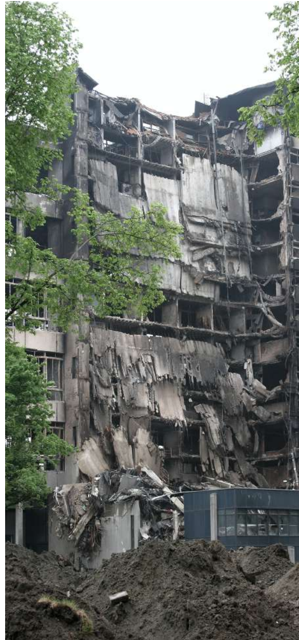
Figure 12: Post-fire collapse of Faculty of Architecture Building, Delft University of Technology, 2008
