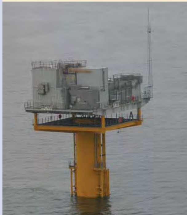
FIGURE B1.16: SUBSTATION AT BARROW OFFSHORE WIND FARM
