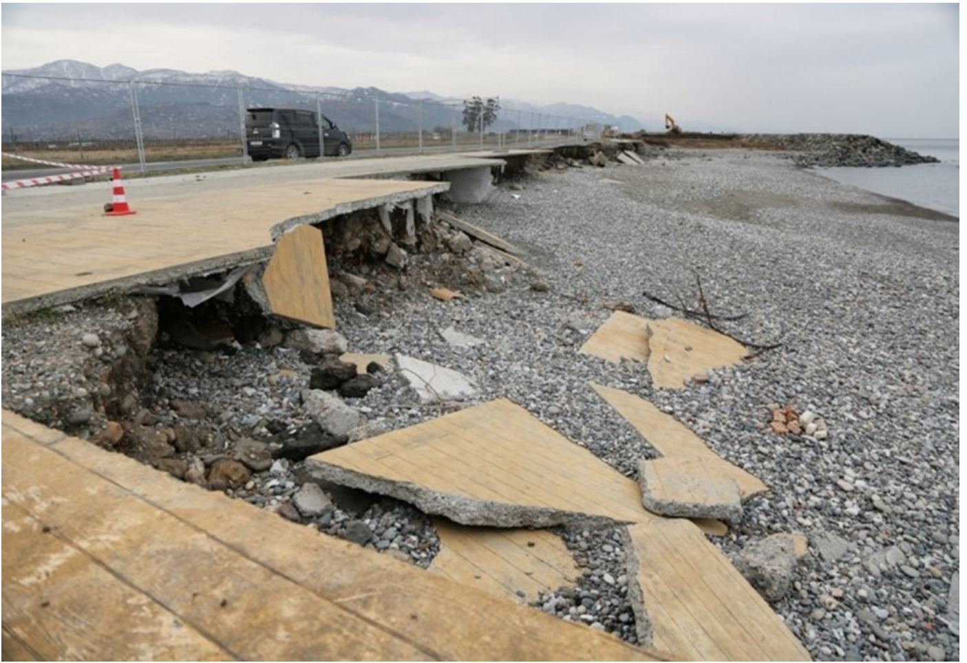
Damage to Batumi boulevard from heavy waves.
