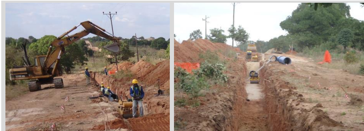
Figure 4-2: Civil works for a transmission main: Space required for safe operation of machines (top) and similar work in confined space using manual labour (bottom), Nampula City.
