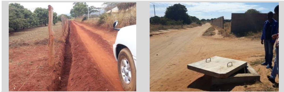
Figure 4-4: Distribution network expansion and maintenance, respectively in Chimoio (left) and Pemba (right)
