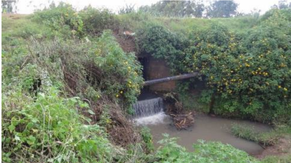
Photo 1-13: Water pipeline on LHS at km 40.6 located in front of culvert end structure
