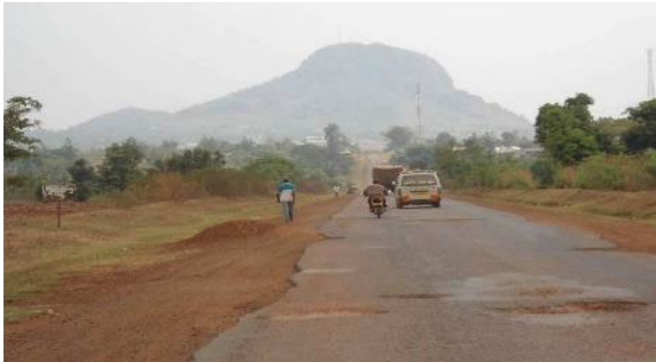
Photo 1-1: Lot 1, Km 7, March 2012, deteriorated section near Tororo
