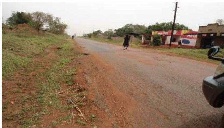
Photo 1-12: Distressed pavement section between Kamdini and Gulu
