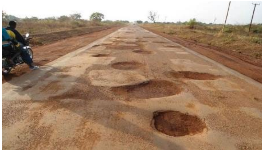
Photo 1-2: Lot 1, Km 104, March 2012, badly potholed section near Kumi
