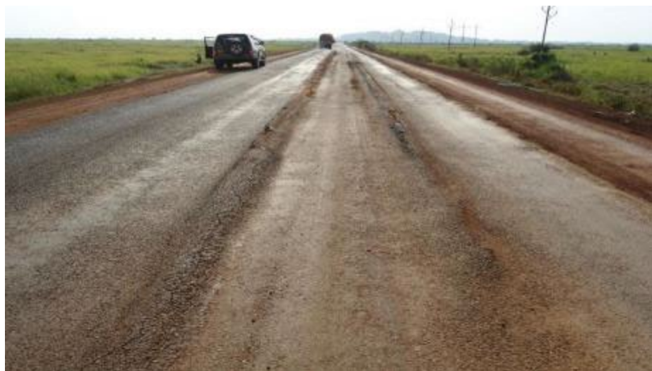
Photo 1-3: Lot 1, Km 132, March 2012: Heaving & rutting Awoja swamp
