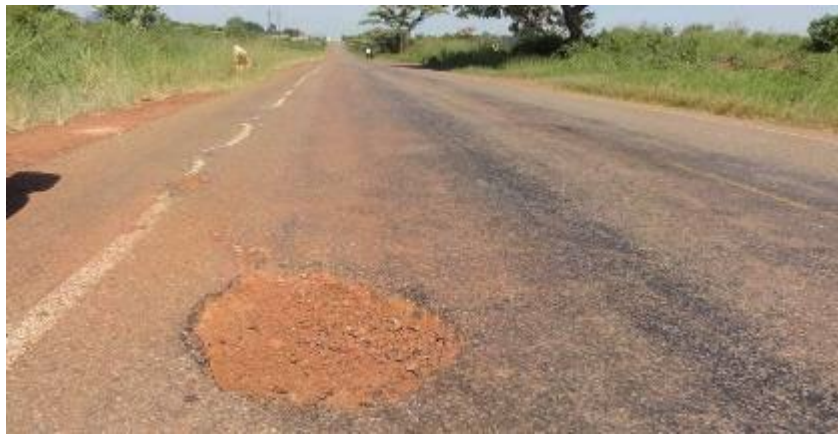
Photo 1-11: Lot 3, Km 41: Potholed and deformed section between Lira and Kamdini
