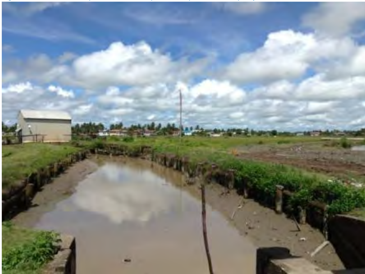
Figure 4.2: Enmore Pump Station. There is potential impact on water quality in this case
