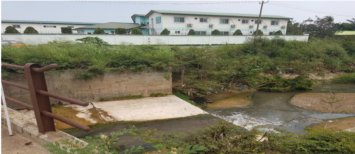
Tema Community 6 drain showing a section to the right where the drain will be lined
