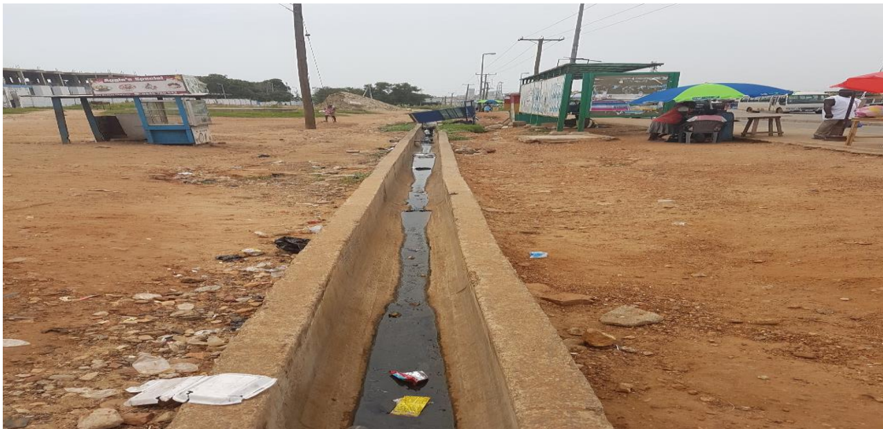
Section of undersized drain in Naval base area which will be reconstructed under the project
