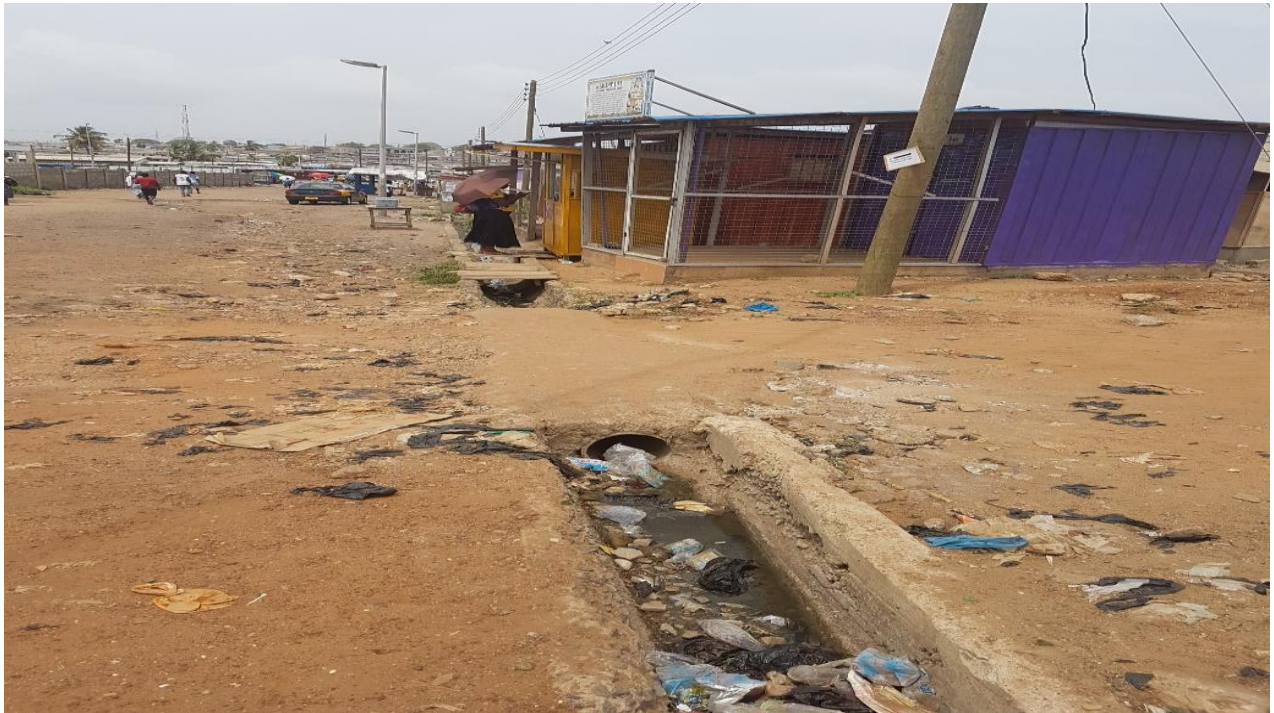
Section of undersized drains at Naval Base area which will be demolished and reconstructed
