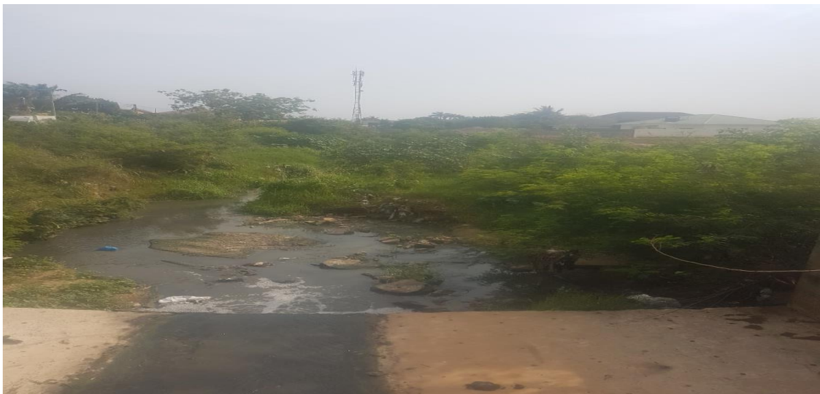
Drain channel at Tema Community 6 that will be lined by the project
