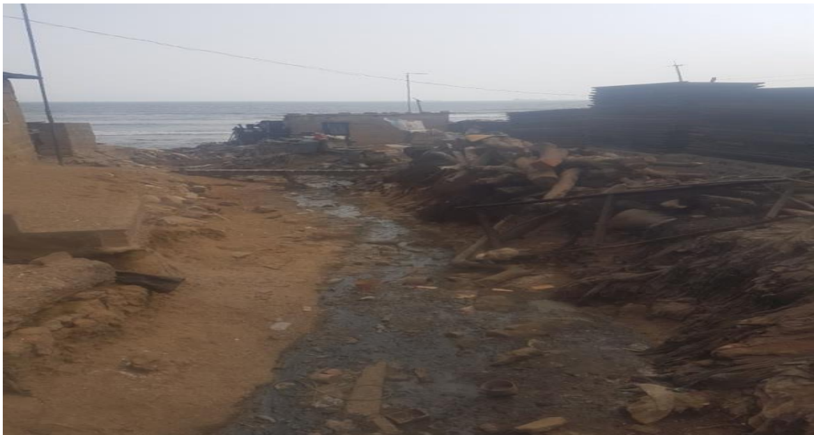
Earth drain course in Bankuman which will be constructed into a drain covered with slap.
