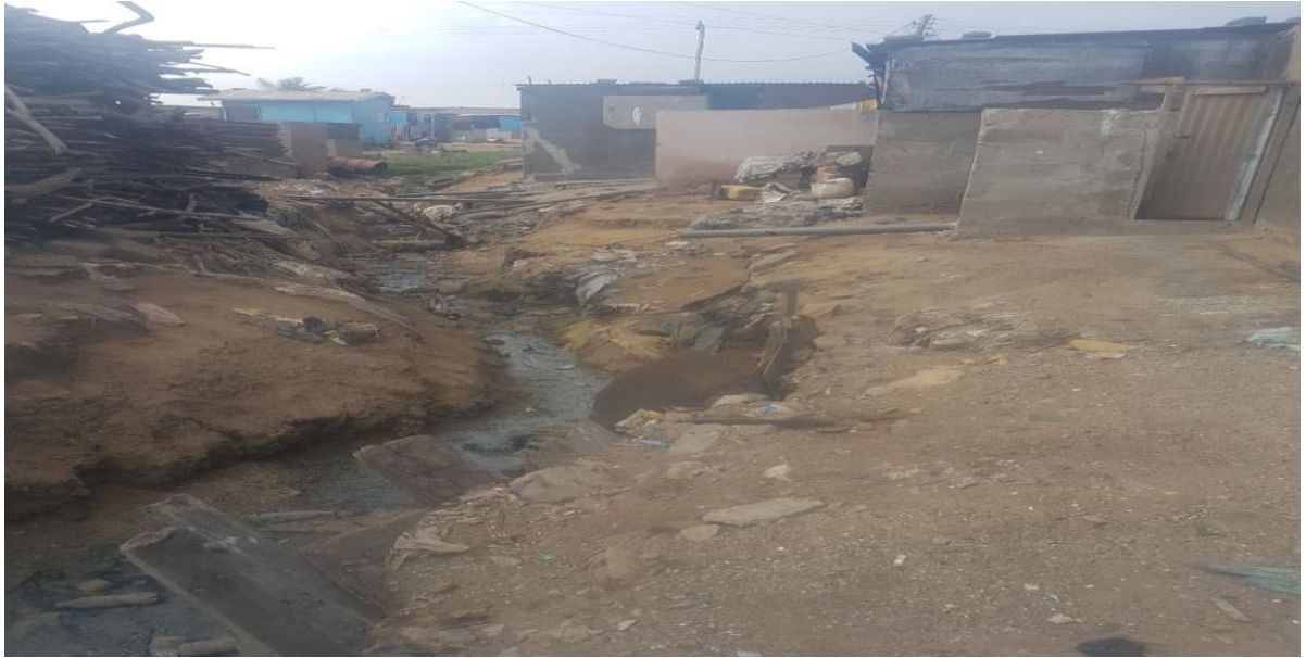
The earth drainage course where drains will be constructed and slapped in Bankuman
