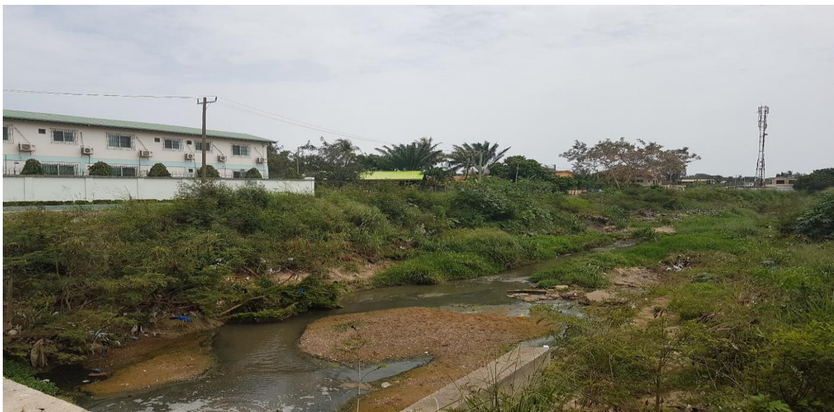
Tema Community 6 drain showing a section to the right where the drain will be lined
