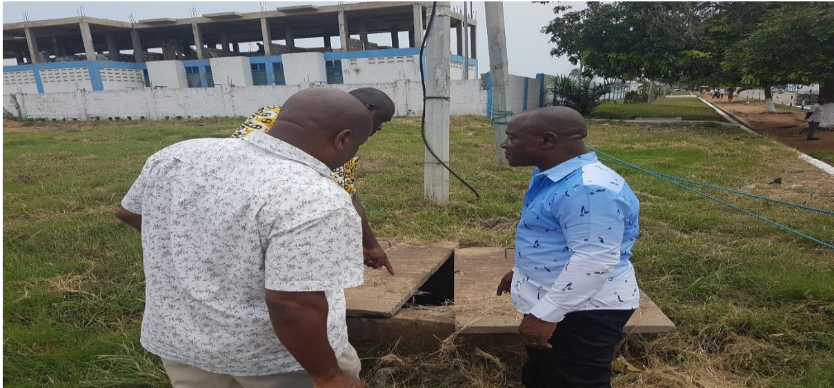
Section of Naval Base area proposed drain site where a GWCL chamber currently exists
