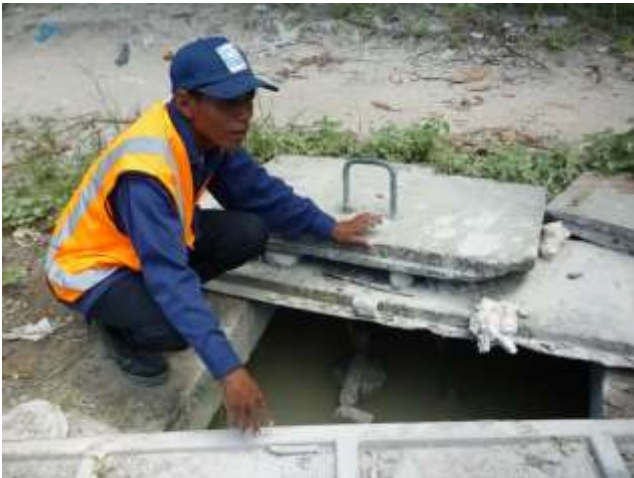
Project-funded Leak Detection Advisor to PUB inspects a valve box (Bikenibeu)
