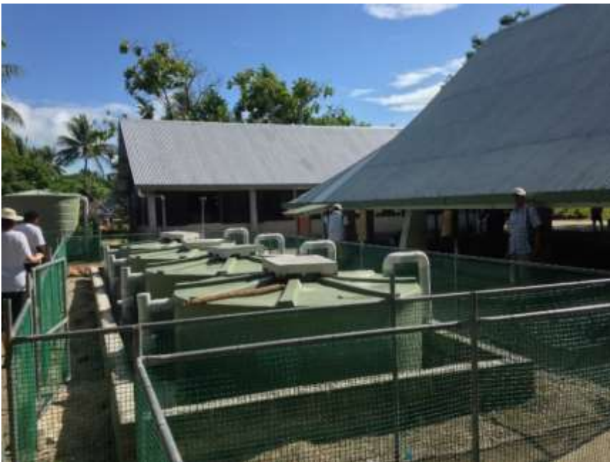
Water storage tanks as part of the Tabonibara rainwater harvesting system in North Tarawa. Water is collected from the roof of the adjacent maneabwa.
