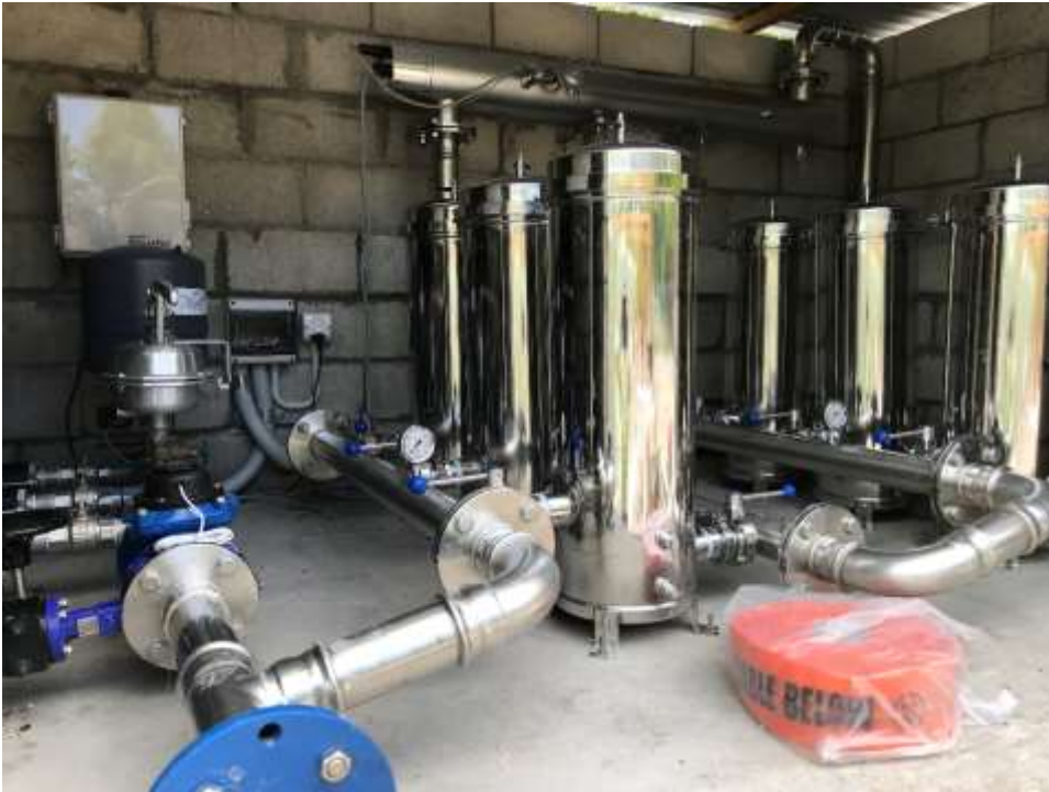
Treatment system for Buota rainwater harvesting facility.
