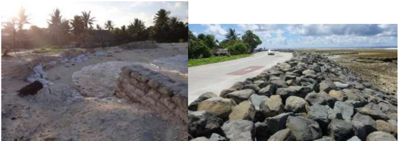
Coastal protection works at Site 10 in Temaiku designed and construction funded under KAP III (by the KRRP civil works contractor). Left: before showing erosion and diversion of road; Right: completed works designed for a 50 year return period event with sea level rise.
