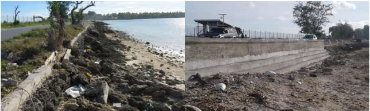
Coastal protection works at Site 2 (Nanikai—Tearaereke causeway). Left: before showing breaches in existing wall; Right: nearly completed gravity concrete wall before reinstating the beach.
