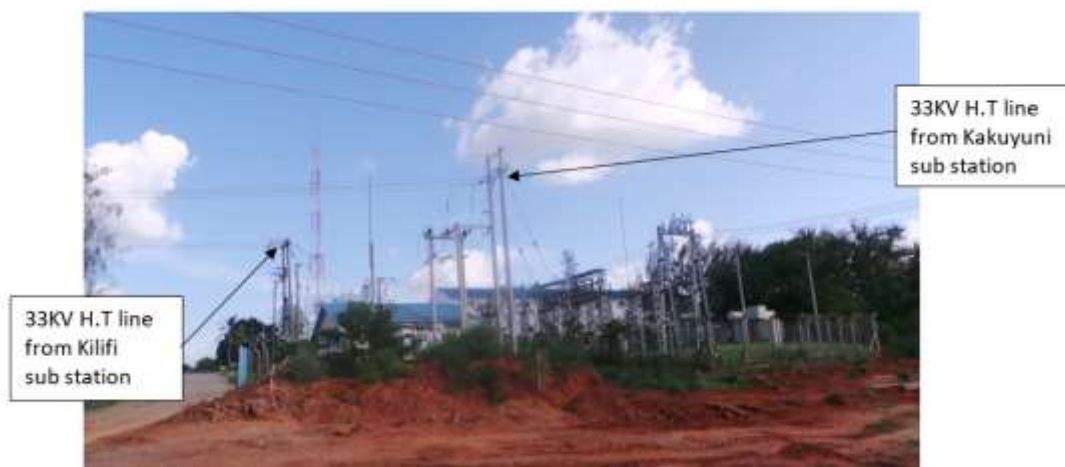
Figure 2-5: Baricho Water Works 33KV overhead H.T lines and substation
