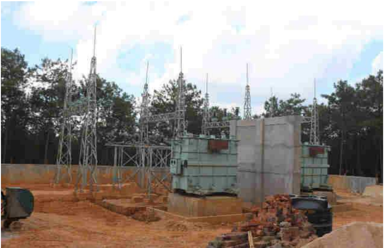
Site Visit to 33/11kV New Shillong
