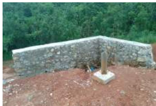
Plate- 5.10 Revetment Wall provided for Tower Protection in 220 kV D/c Byrnihat-Mawngap-New Shillong
