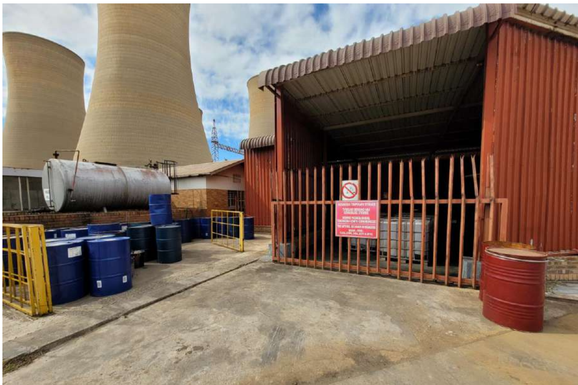
Figure 98: Hazardous substances storage area
