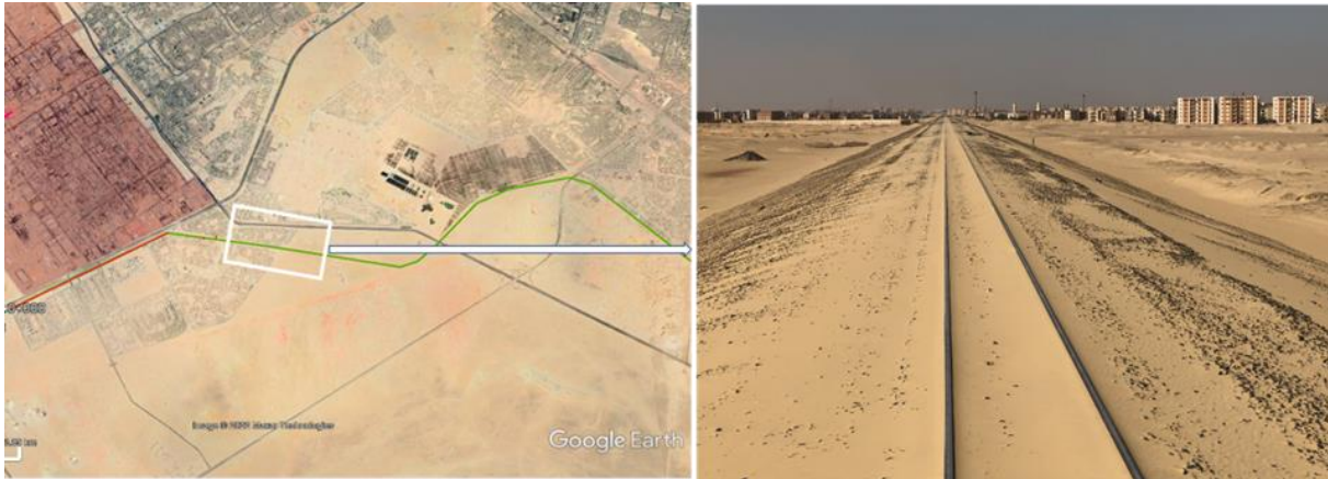
Figure 4-42: Buried sleepers and tracks under sand
