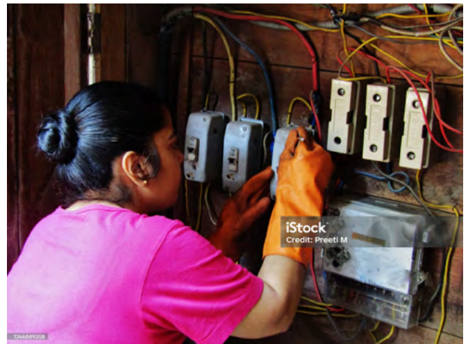
Female electrician checking power. © Preeti M
