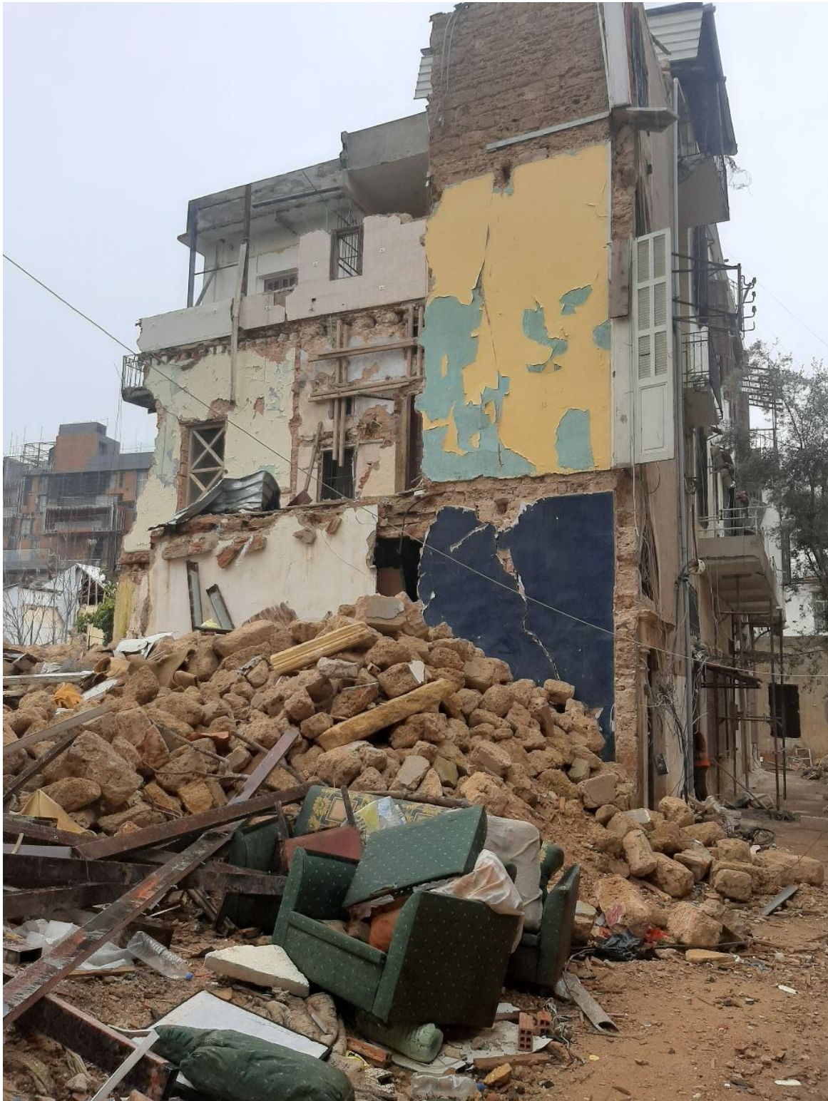
Figure 2. Example of a building with level 4 damage
