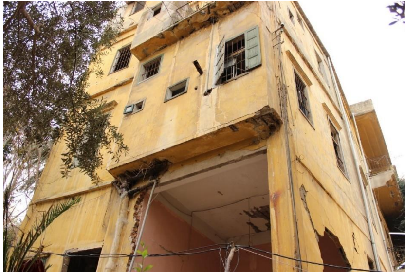
Figure 3. Example of a building damaged by the POB
