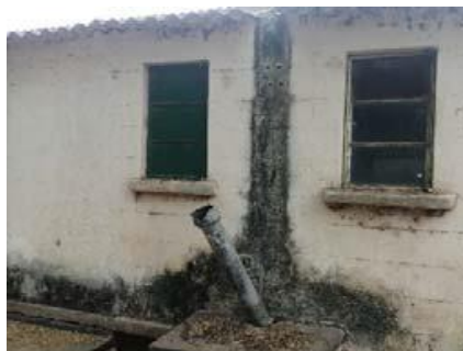
Figure 2. Asbestos in plumbing pipework
