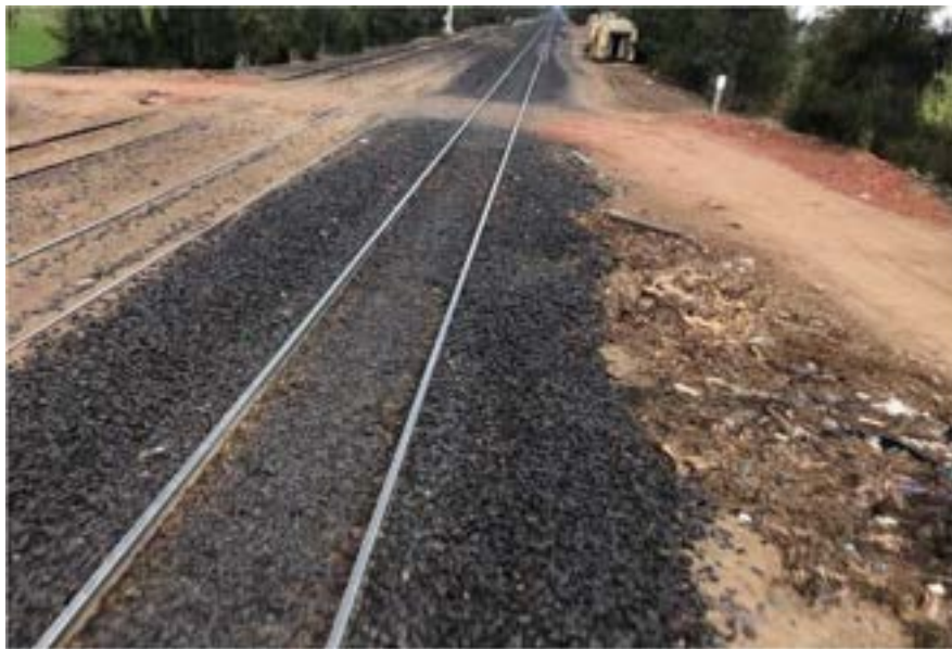
Figure 4-31 illegal level crossing for vehicle
