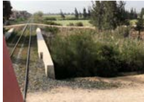
Very Narrow bridge crosses the watercourse and Illegal level crossing
