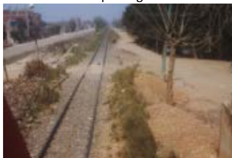
Illegal level crossing
