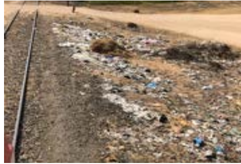
Solid wastes and illegal level crossing
