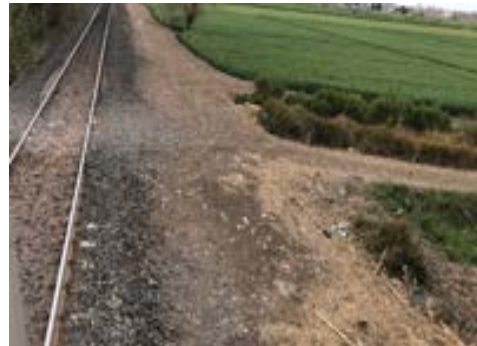
Illegal level crossing
