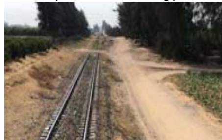
Illegal level crossing between agricultural lands
