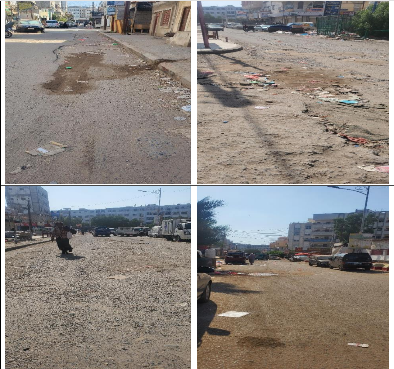
Stone paving for Street extending from intersection of Shamsan Mall with Ghurairy restaurant to Abdullaziz Area - Sheikh Othman District
