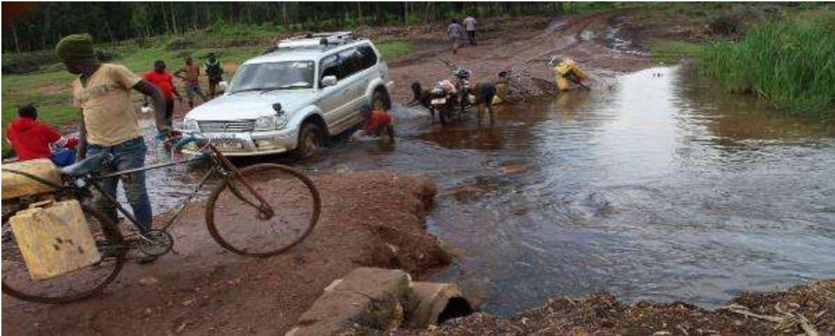
Figure 4-65: Poor road and river stream used as water sources in the irrigable area at237333, 9895668
