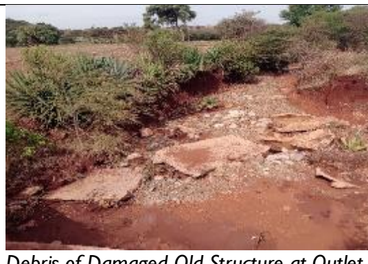
Debris of Damaged Old Structure at Outlet End of Box Culvert at Ch. 78+470
