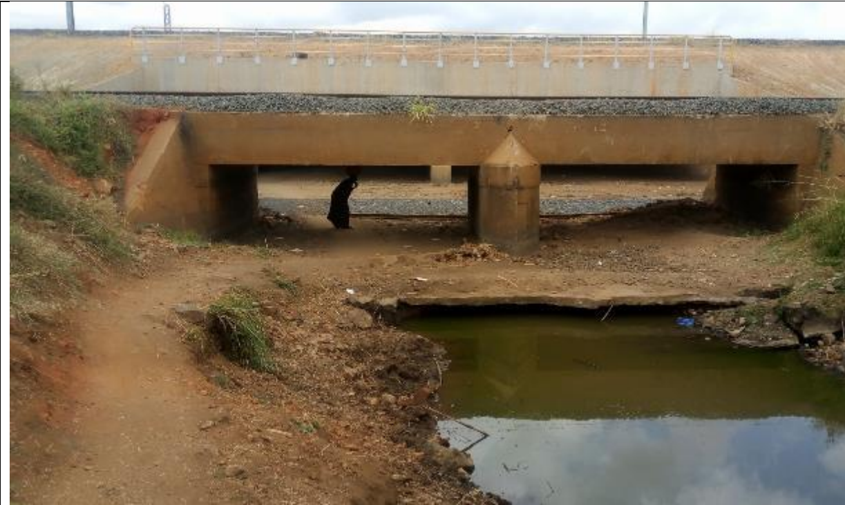
Ponding/Stagnation of Water at Chanzulu Bridge at Chainage 273 +390
