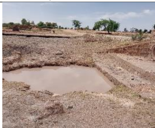
Scour Hole at Outlet End of Pipe Culvert at Ch. 50+786
