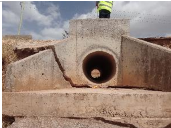
Damaged End-Structures of CPC 900 mm at Ch. 1+490
