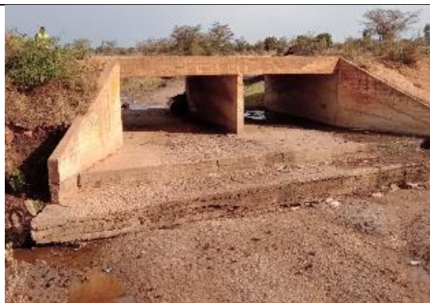
Outlet End of Box Culvert at Ch. 44+625. Eroded behind Wing walls
