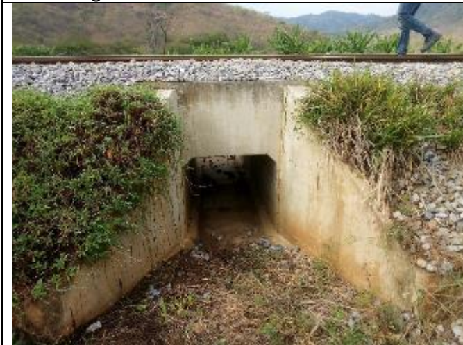
New CBC Structure constructed in the recent TIRP I Improvements at Munisagara (Kilosa) at Chainage 295 + 845
