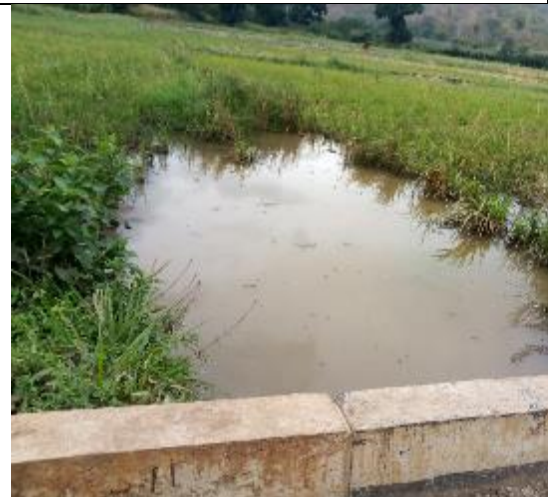
Ponding/Stagnation of Water at Outlet of a Small Slab Bridge at Chainage 296 + 210
