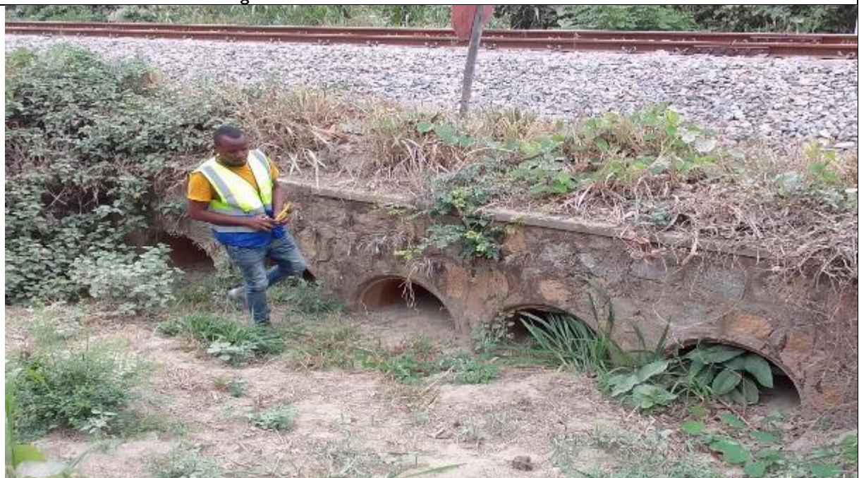
Over 50% Clogging of 5 cells of CPCs at Mkadage (Kilosa) at Chainage 284 + 050
