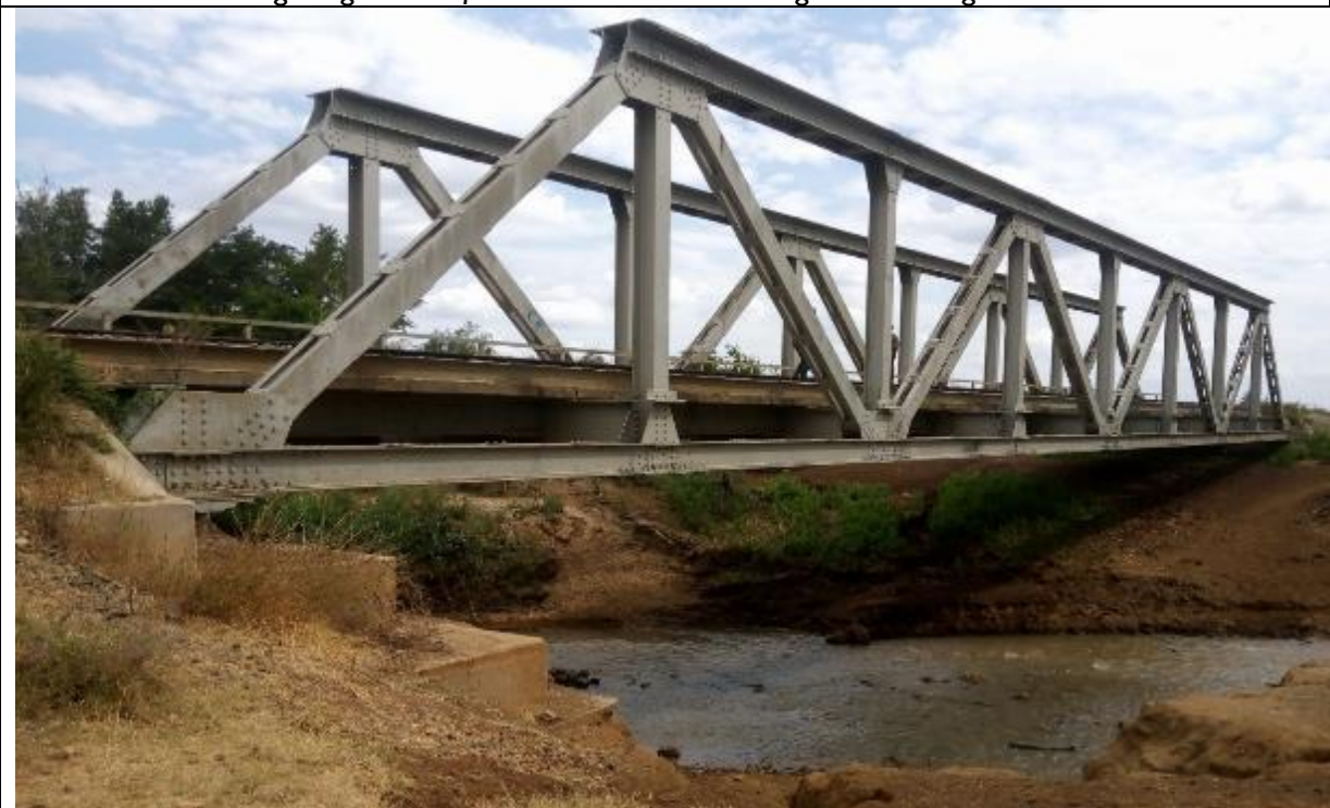
Downstream of the Main Mkata River Bridge at Mkata (between Kilosa and Mvomero).
