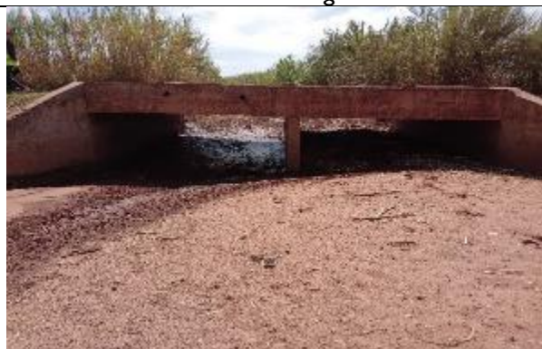
Severe Siltation of Box Culvert at Ch. 64+081
