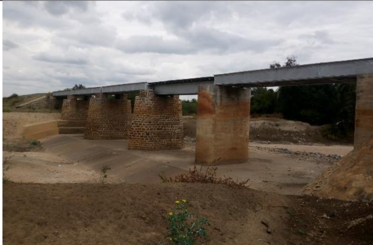
Downstream of a Minor Mkata River Bridge at Mkata (between Kilosa and Mvomero). at Chainage 293 + 707
