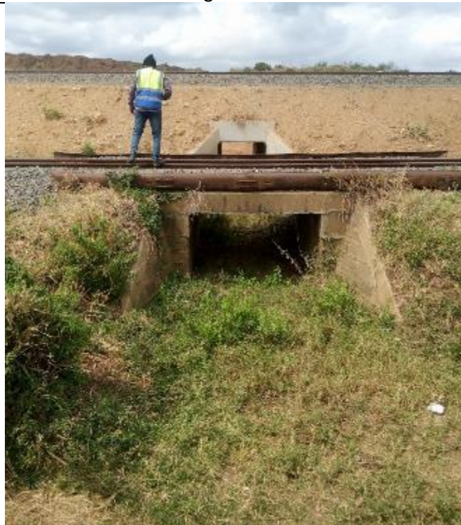
Proximity between MGR and SGR Tracks and Drainage Structure dominant at Chanzulu (Kilosa). at Chainage 274 +634
