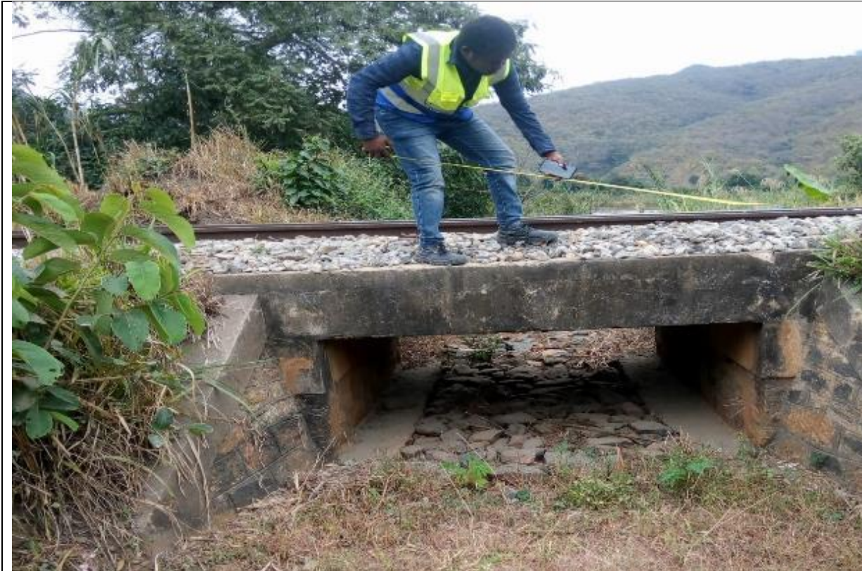
Inadequate/insufficient opening sizes led to severe overtopping of the railway track at the Munisagara plain (Kilosa). It was noted that, 3 years ago, the Mkondoa River spread greatly, resulting in flooding. at Chainage 300 + 883
