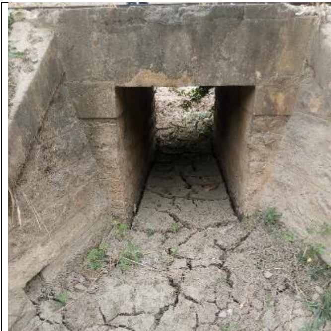
Soil Deposition inside opening of a Small Box Culvert at Mzaganza (Kilosa) at Chainage 305 + 509.6
