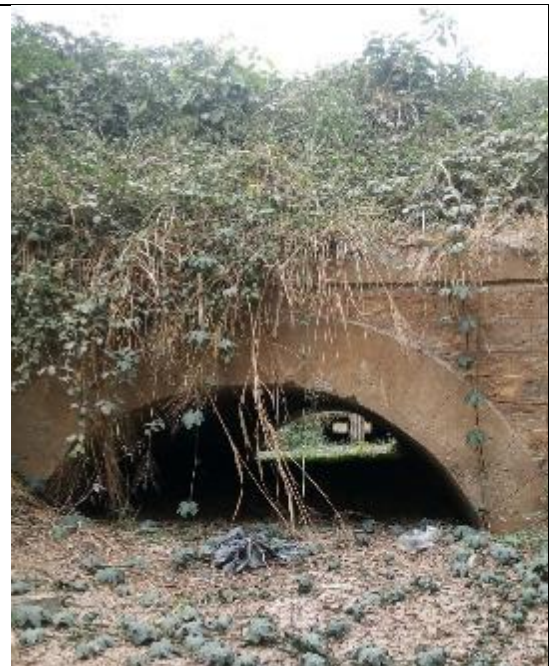
Nearly 70% of anticipated Opening Size is clogged with Sand/Siltation at Mzaganza (Kilosa) at Chainage 305 + 146
