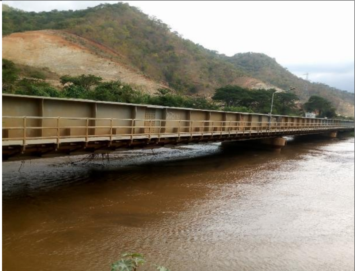
Upstream of the great Mkondoa River Bridge at Munisagara (Kilosa). Water is known to reach the Steel Girder Level at Chainage 294 + 371
