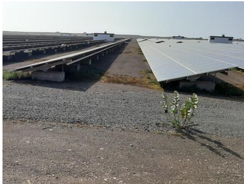
Photo 2 - Solar PV panels and support structure set in concrete blocks (Sal Island)
