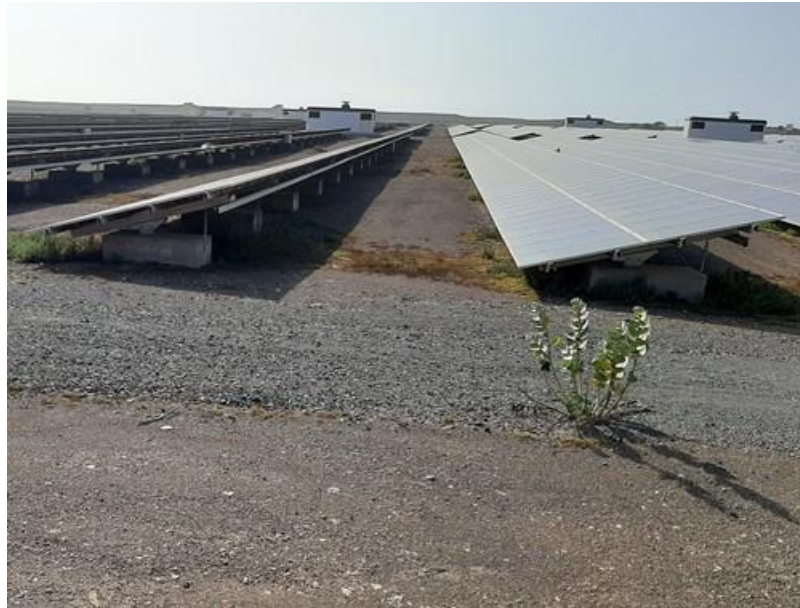
Photo 1 - Solar PV panels and support structure set in concrete blocks (Sal Island)
