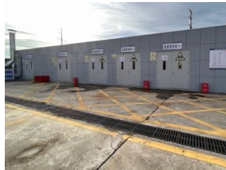
Fig 6: Hazardous waste storage rooms at YWSVDC
