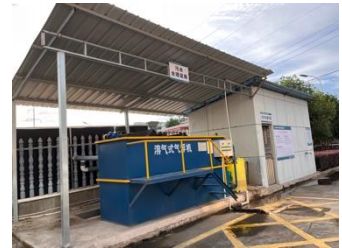
Fig 7: Wastewater treatment facilities at YWSVDC
