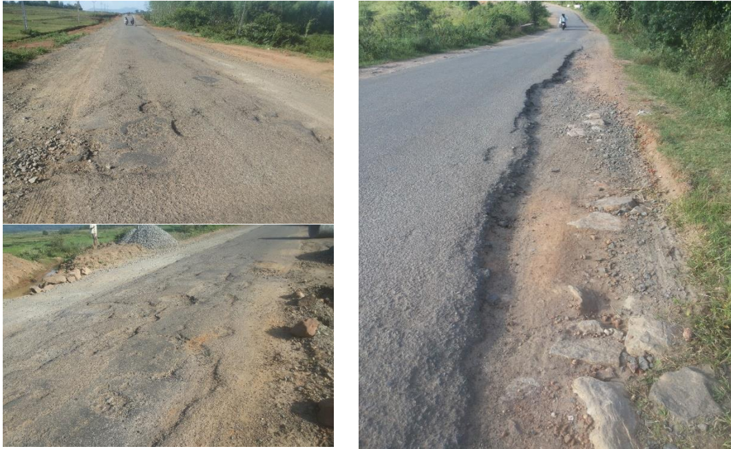
Figure 0.3: Pavement Condition of the Project Road
