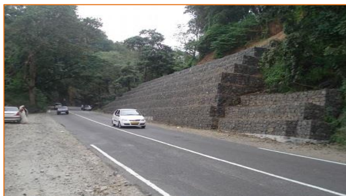
Figure Error! No text of specified style in document..6: Gabion Walls for Slope Protection
